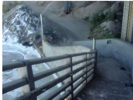
Stairs at end of pathway - closed off
