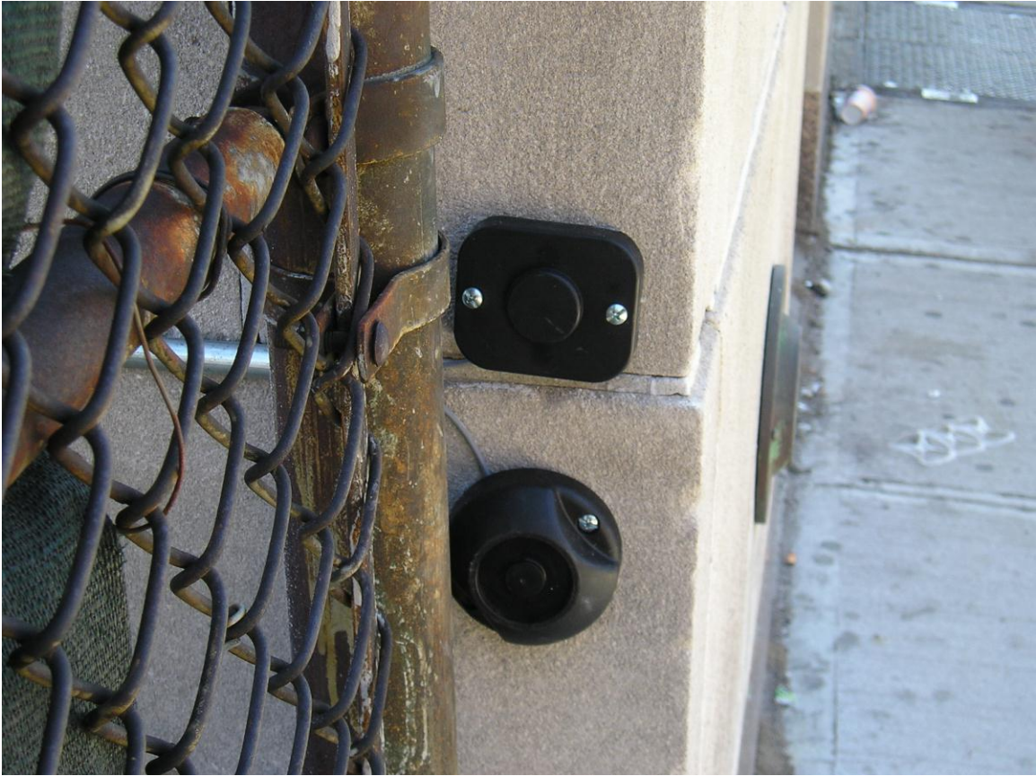
Figure 1 Meter Remote Pads (No Longer Used by DEP)
