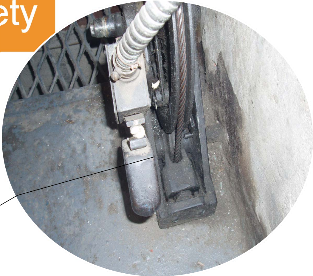
Governor switch blocked
