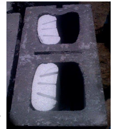
Insulation inserts within CMUs - No Credit allowed in R-Value Method (Use U-Factor Alternative)
