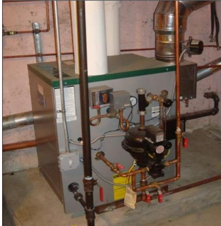
Photo: Courtesy of energy.gov
