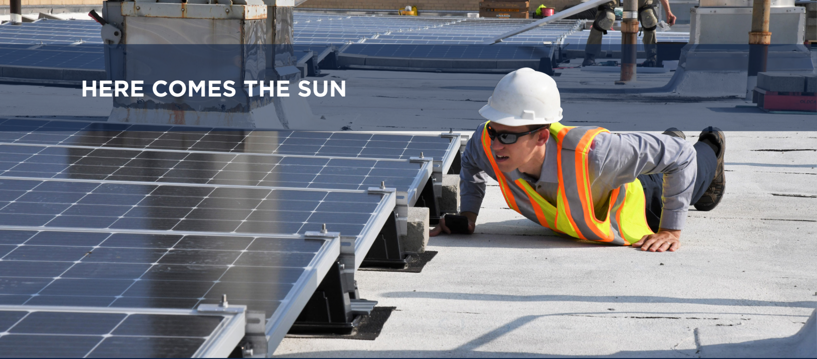
DEM Project Manager Dylan Roller monitors the installation of new solar photovoltaic panels at the Adrien Block School I.S. 25 in Flushing, Queens.
