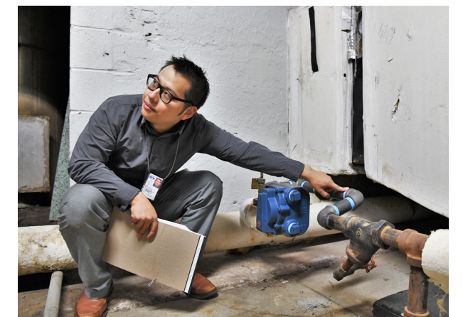
Lin reviews the replaced Float and Thermostatic steam trap to make sure the contractor installed the correct size.
