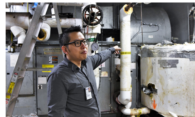
Pointing to the repaired air handling unit, Deng Lin, Deputy Director of the Technical Services Team in DCAS's Division of Energy Management, explains its new sequence of operations.
