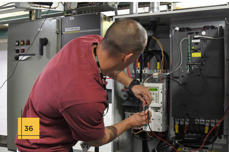
Chris Keddy, Controls Specialist for DCAS's Maintenance Collaborative Group, installs a Variable Frequency Drive (VFD) to 111 Centre Street's HVAC system. The VFD allows for greater control of air conditioning through the building so that heating and cooling only occurs when necessary.
