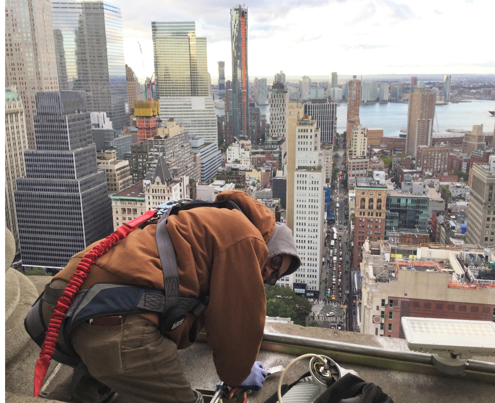
DCAS Electrician Nyron Ali installs light fixtures on the ledge of the building.
