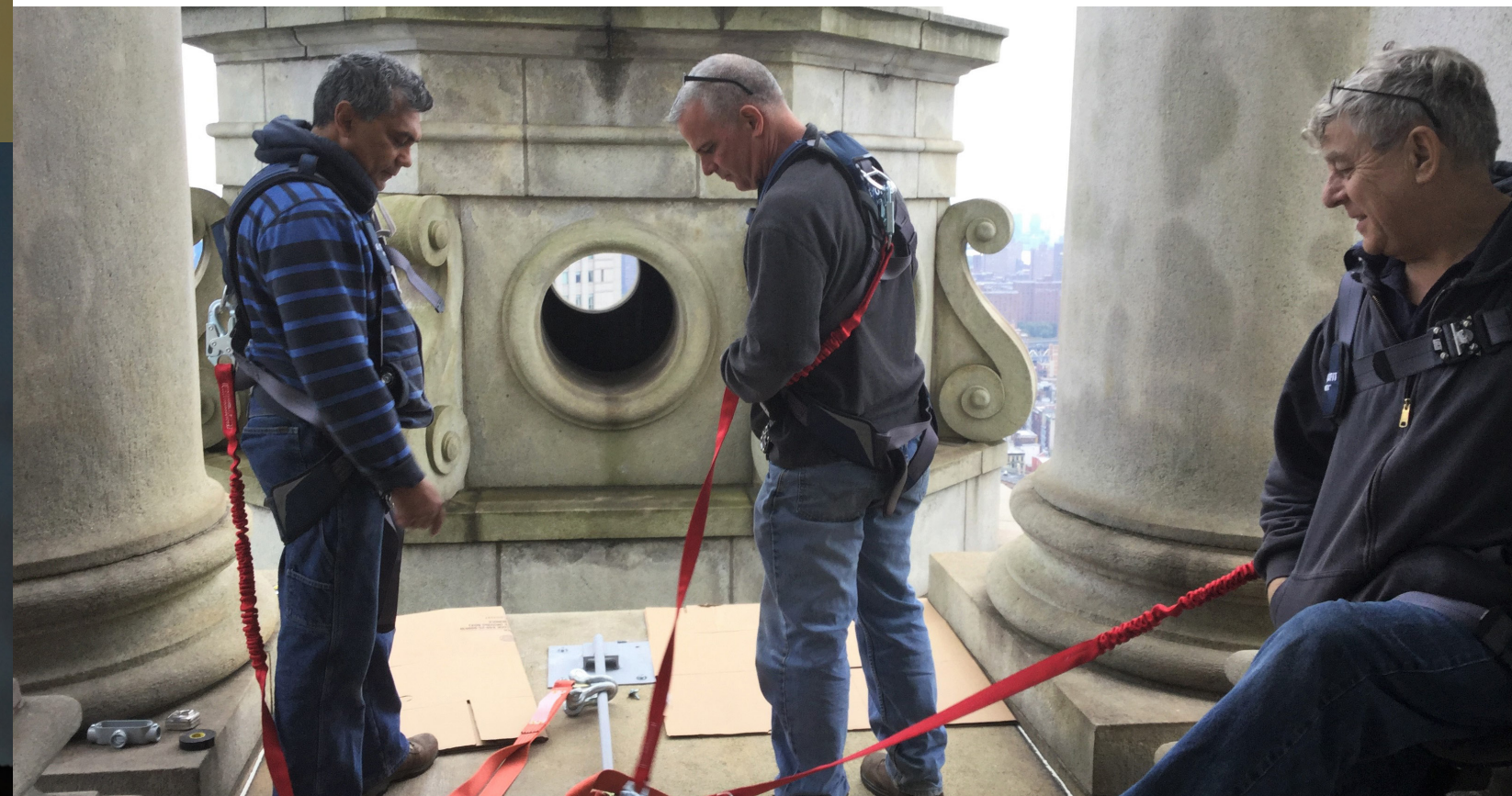
Nyron Ali (left), Steve Carlucci (center), and Leszek Beksinski, the lead electrician (right), all from the DCAS electrical shop, harness up to go on the building's ledge to install the tower's new light fixtures.
