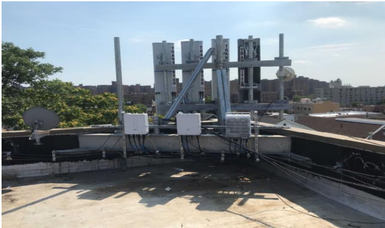
Figure 12. A steel flange support at a corner parapet that counts toward “related cellular equipment”.
